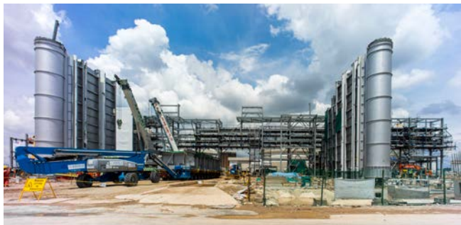
Photo: Construction progressed on a cogeneration plant at the Singapore Refining Company.
