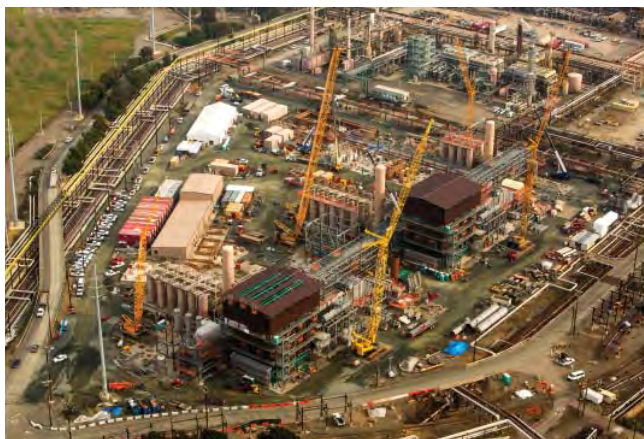
Photo: Field construction activity restarted during 2016 for the modernization project at the company's refinery in Richmond, California.
