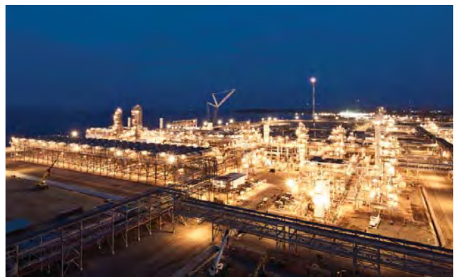
Photo: During 2016, production restarted and LNG cargos resumed at the Angola LNG Plant in Soyo, Angola.
