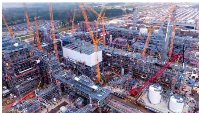
Photo: Construction activities continued during 2016 at CPCChem's U.S. Gulf Coast Petrochemicals Project in Texas.
