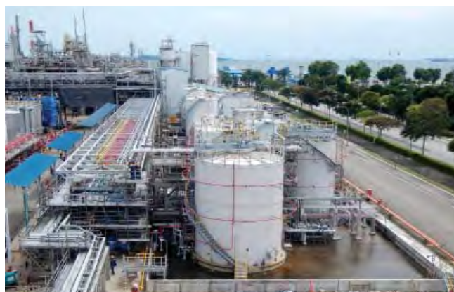
Photo: Construction progressed on a new carboxylate plant at the company's additives plant in Singapore.
