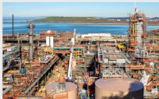
Photo: The Richmond refinery modernization project is designed to improve reliability.
