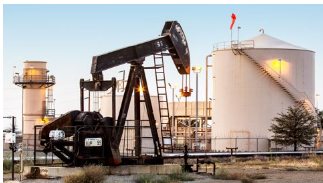
Photo: A pumpjack near a cogeneration power plant in Coalinga, California.
